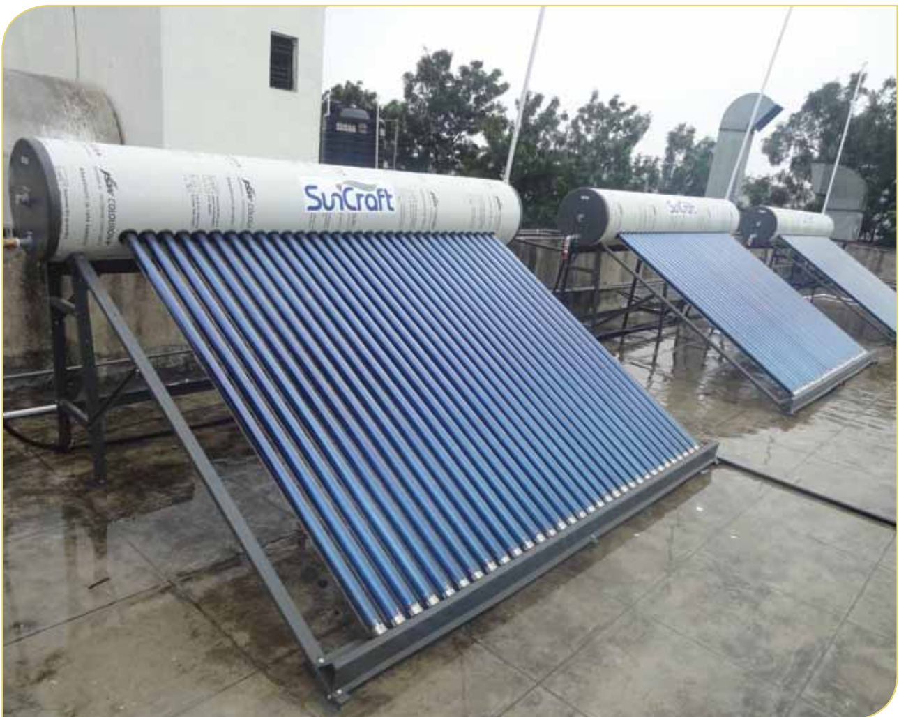
Solar Water Heater at the Rooftop
