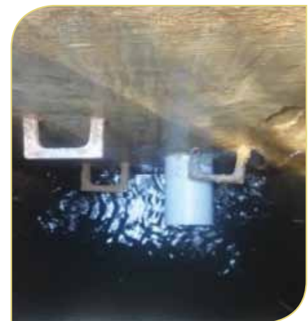
Water Harvesting Tank at MSIL Pune
