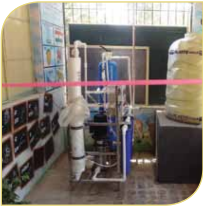
2 units of RO Plant Inaugurated at Pune on 14th April 2017
